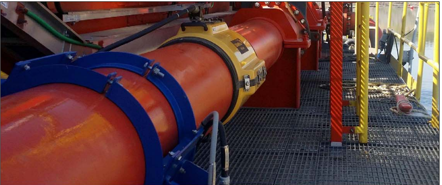
The brass-toned meter (i.e., SONARtrac meter) installed on a working dredge discharge pipe.
