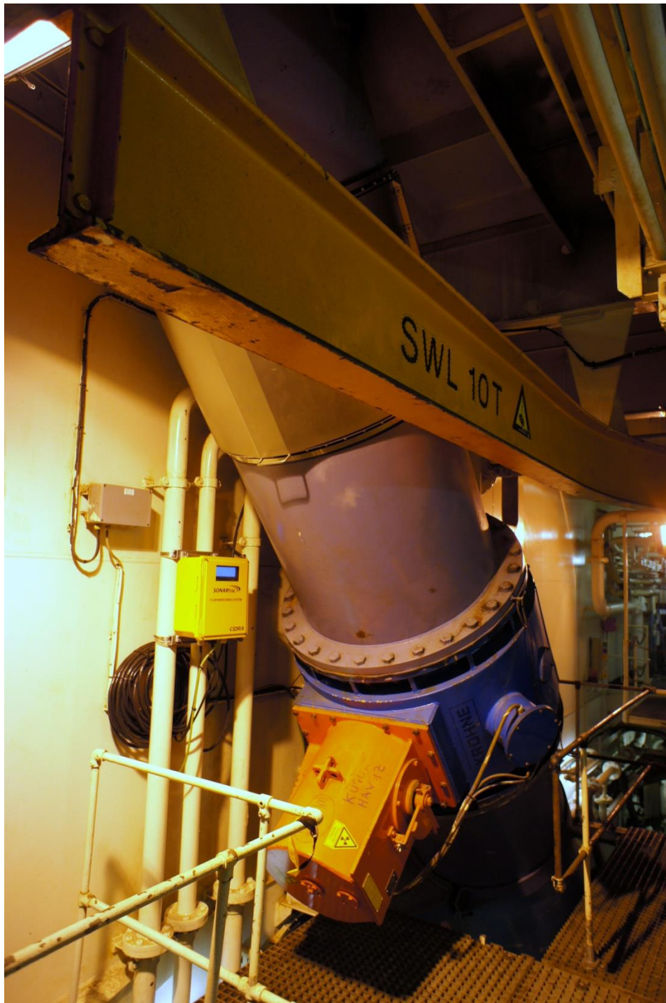
Figure 2. Photograph of the sonar based flow meter as installed.
