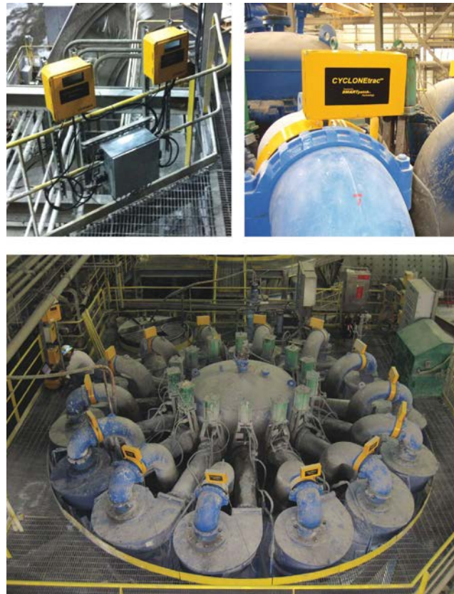
Figure 1 Installed CYCLONetrac OSM System at Kennecott with transmitter and junction box (upper left picture), sensor head (upper right picture), and a completely instrumented hydrocyclone battery (bottom picture)
