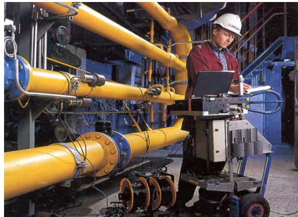
Figure 5 On-site flow calibration on a natural gas line
