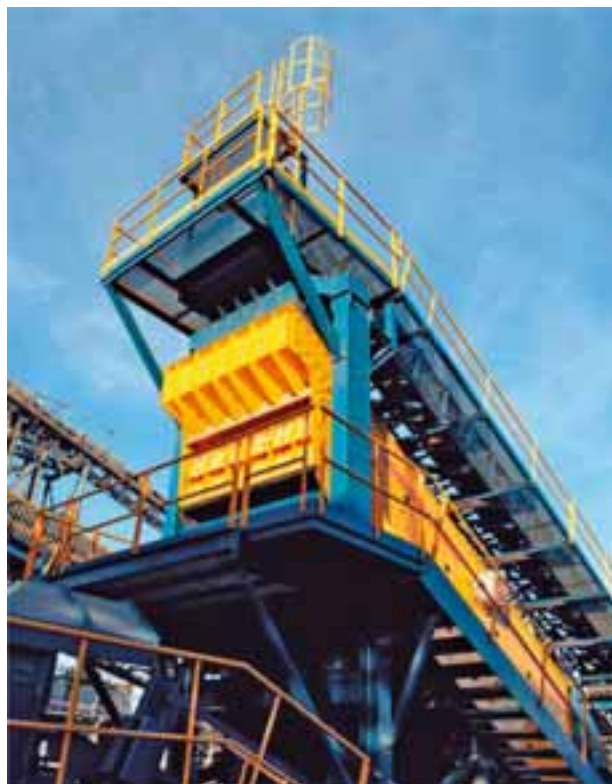
All vibrating equipment at Neves-Corvo, such as this Nordberg TS Series inclined screen from Metso, is painted yellow for safety reasons
