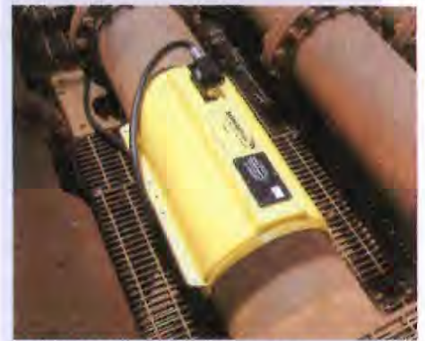
CIDRA slurry flowmeter, Worsley Alumina
