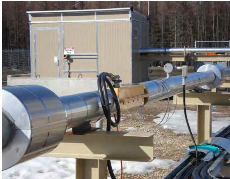
Figure 6: Passive sonar meter installation on water reinjection line
