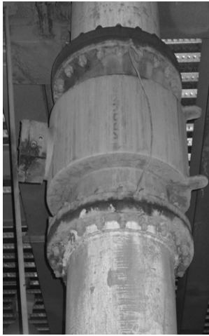
Figure 7 Failed Magmeter with Slurry
