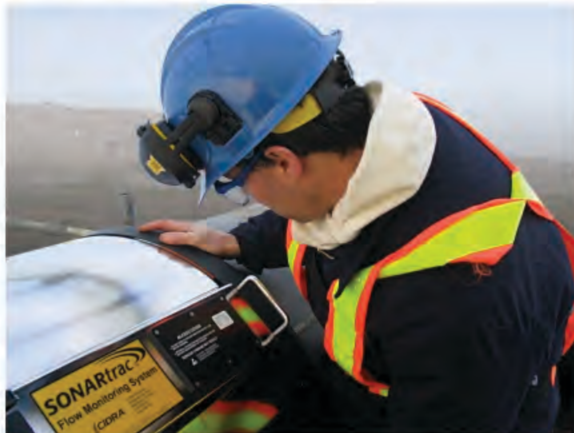
Mark Fernald, VP of Engineering, installing a CiDRA SONARtrac system in the oilsands of Alberta, Canada.
