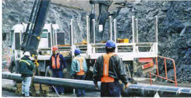
The first multi-product slurry pipeline system in a mountainous region, Antamina was designed for the transportation of a maximum of 1.4 Mt/y of copper and zinc concentrate from the mine, at an elevation of 4,100 m, to terminal facilities at Huarney
